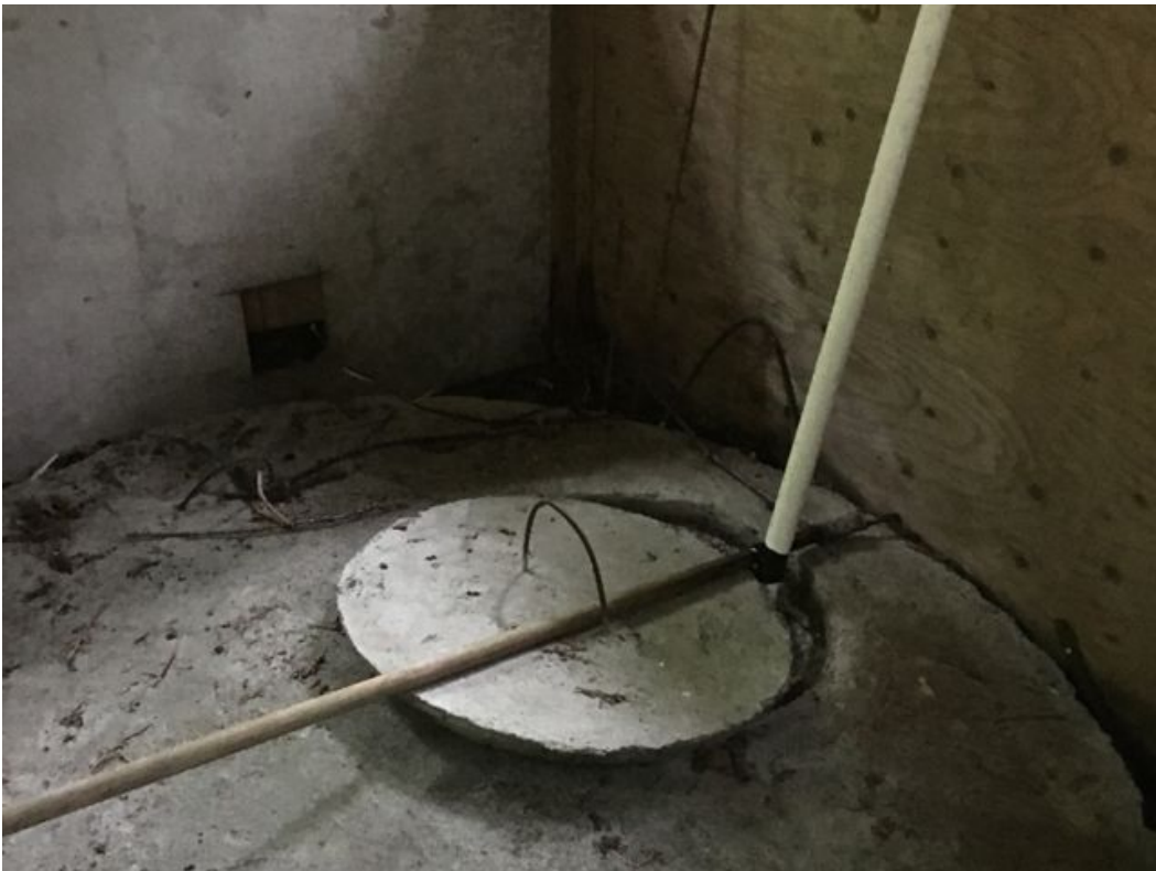
Photo 4, Appendix B. Access cover to Spring A on subject property.
